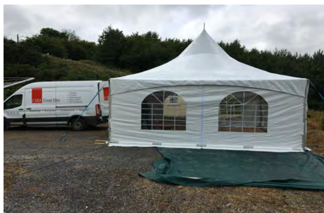
Our 6m x 6m under construction in Innishannon for a home wedding. 40 guests attended. Side-view. Flooring installed. July 2021.
